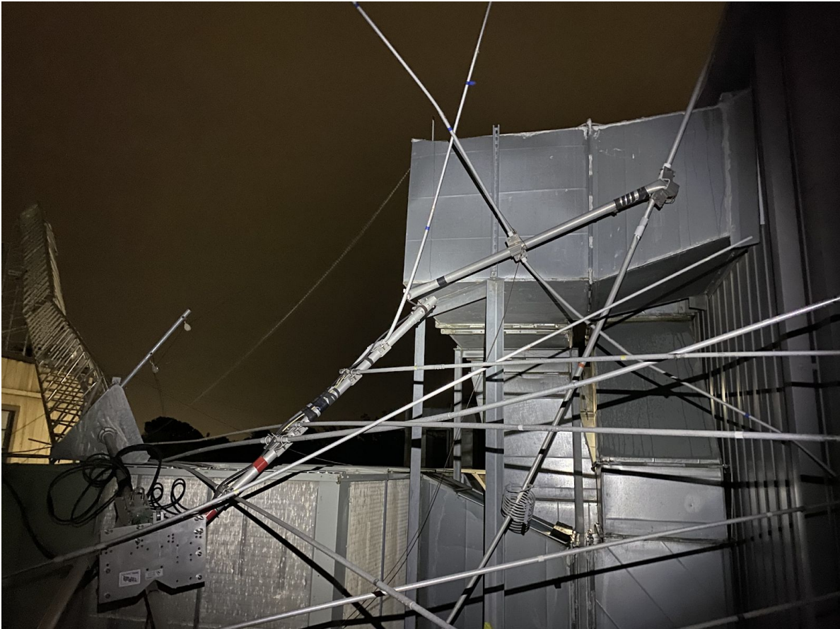
A close-up of damage to the Force 12
