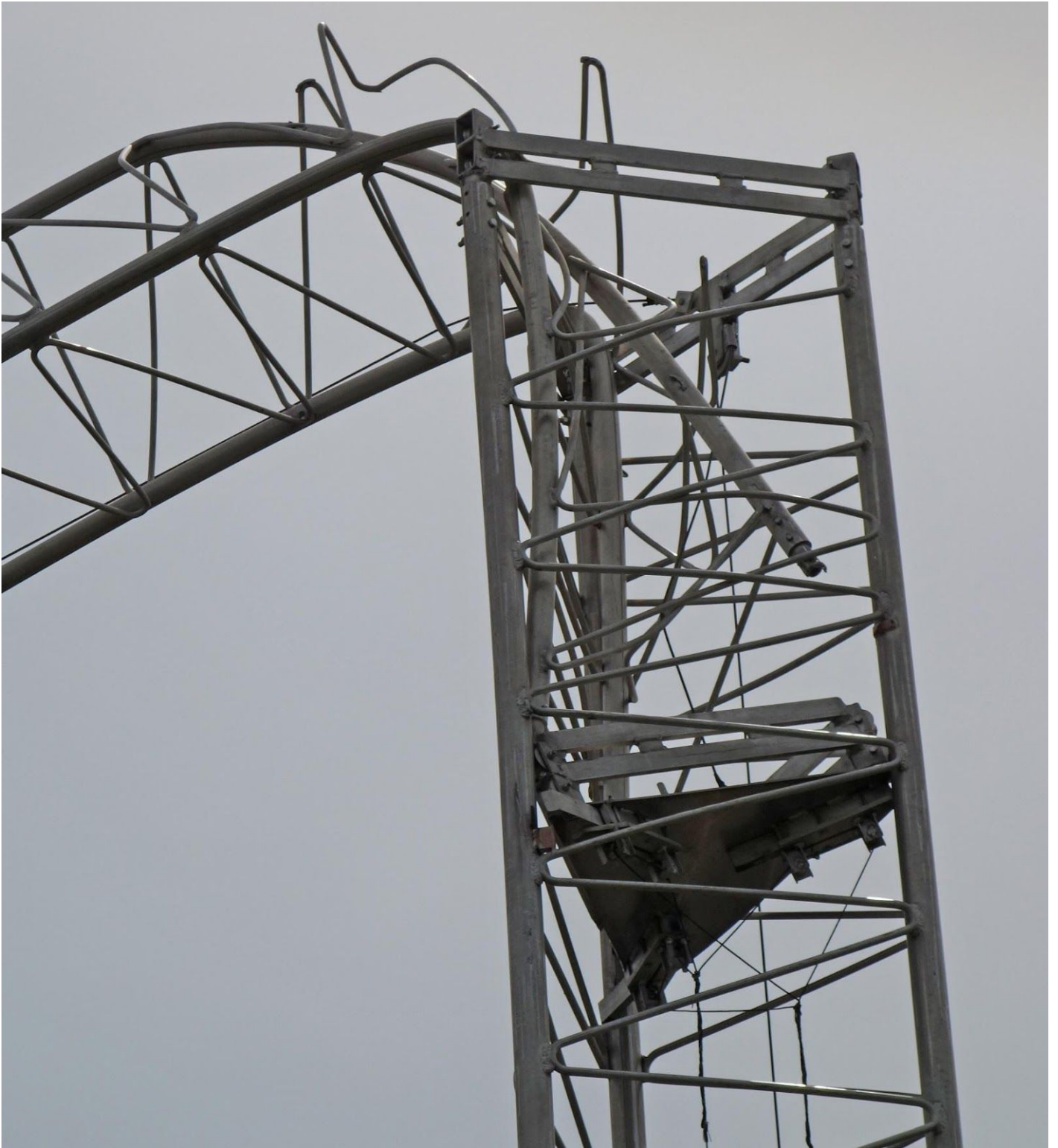
Where the tower failed at the bottom of the second section
